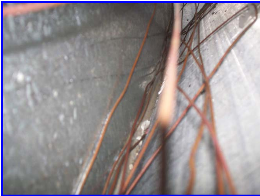
ROOM # 224-VENTILATOR BLOWER
