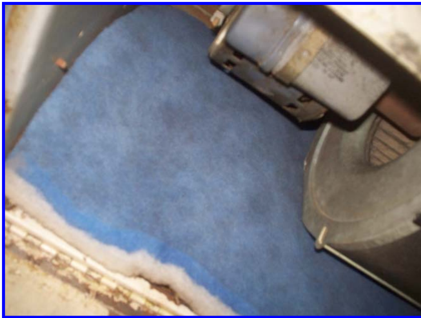
LIBRARY SEMINAR ROOM-UNIT COIL/DRAIN PAN
