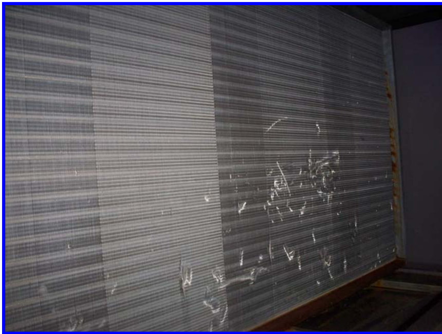
AHU # ?-CAFETERIA -BLOWER
