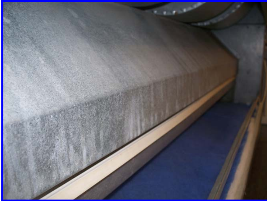
AHU # 3-OFFICE AREA-COIL-CEILING
