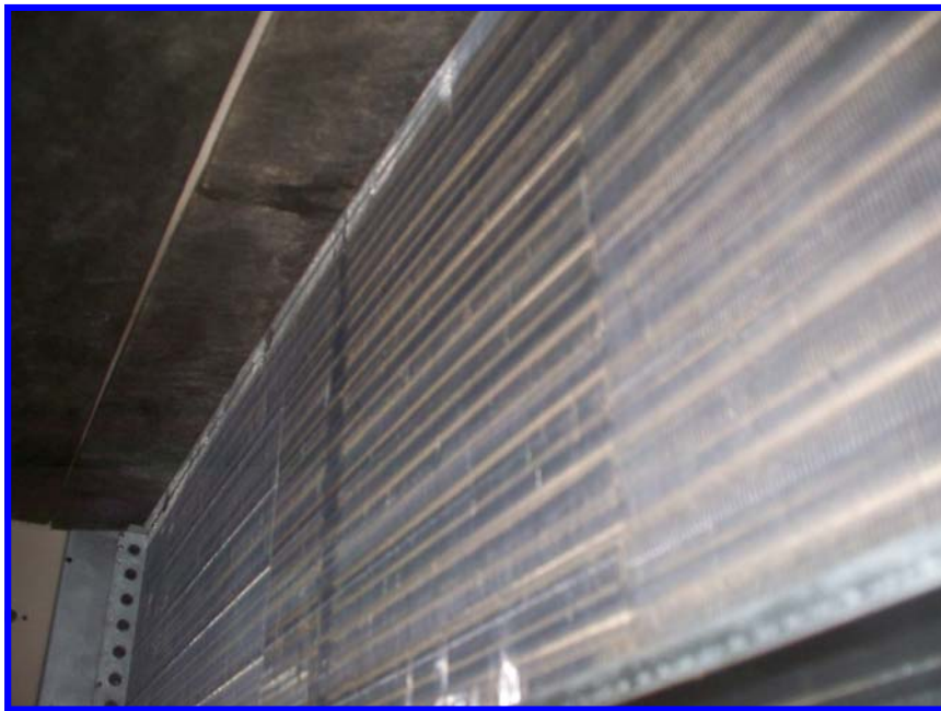
TEAM ROOM-UNIT COILS DOWNSTREAM
