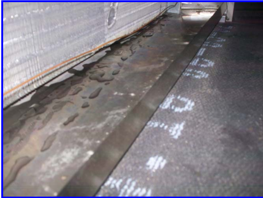
ROOM # 137-UNIT BLOWER
