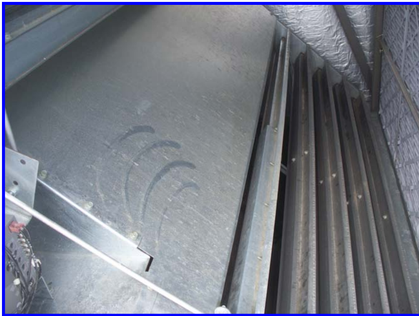
RTU -GYMNASIUM FARTHEST FROM FLAGPOLE –FILTERS
